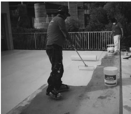
Apply Elastomeric Basecoat ahead of the Fabric at 100 square feet per gallon.
