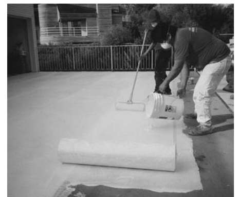
Apply Elastomeric Basecoat on top of the Fabric at 100 square feet per gallon after rolling it several feet and lightly broadcast some #60 silica sand.
