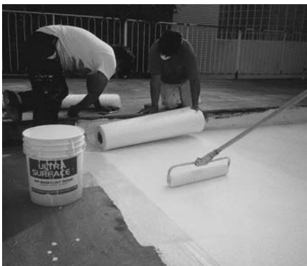
When you reach the end of the deck cut the fabric with a knife or scissors and start laying the next row.
