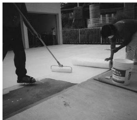
Lay the next row of fabric so it overlaps the edge of the previous row ½ - 3 inches. Continue laying rows of fabric until the whole surface is covered.
