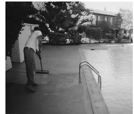
Apply two coats of Colorcoat 100 using a 3/4" nap roller. Option: Apply Sealcoat 1000 clear.
