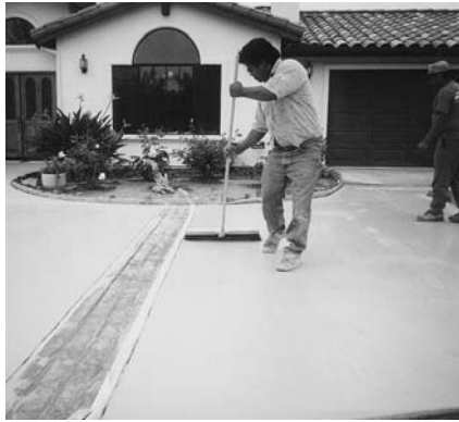
Apply a Fine Broom Finish or Swirl Pattern Finish over the dry Squeeze/Bond Coat.
