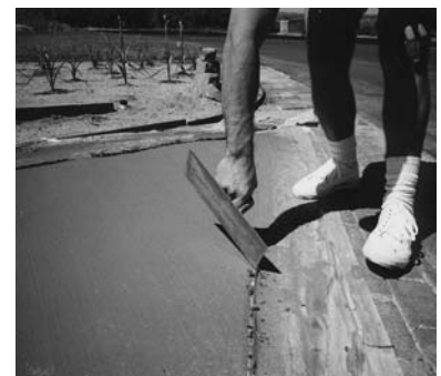
Scrape out any material that got in the joints using a trowel or scraper before it dries.
