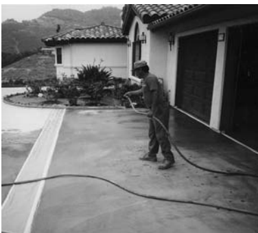
Fog the surface with water where you wish to begin spreading the Squeegee Coat Mix.
